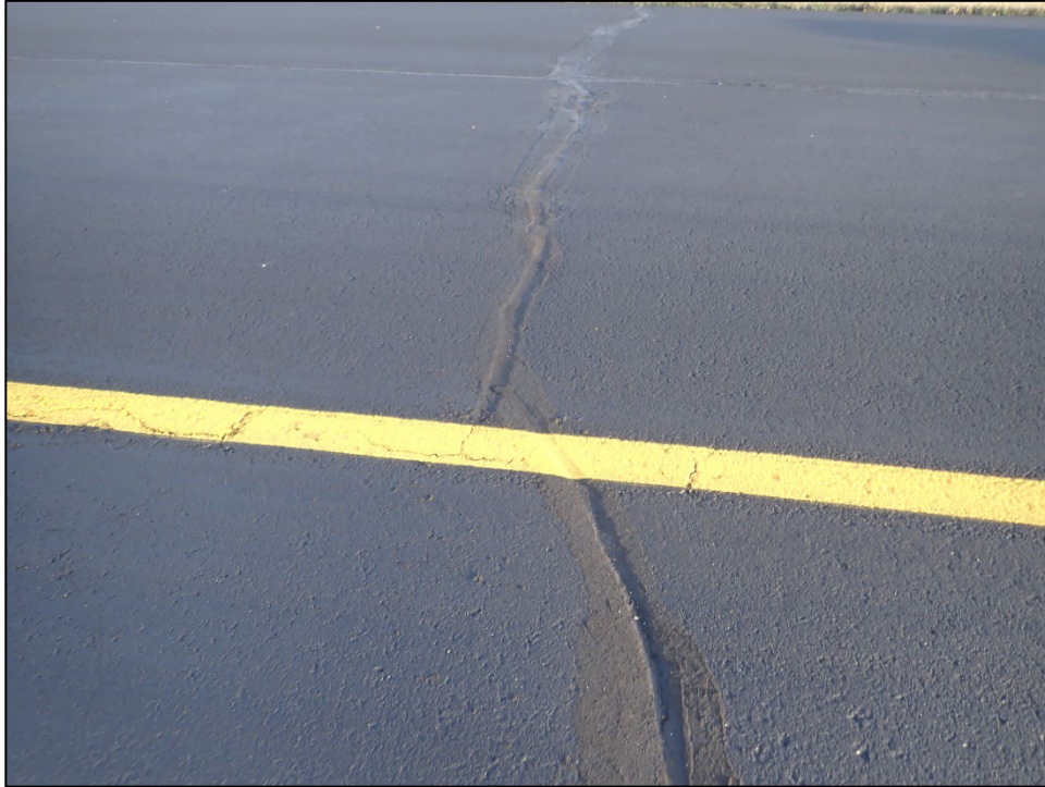
RW04-04-50: L&T Cracking
